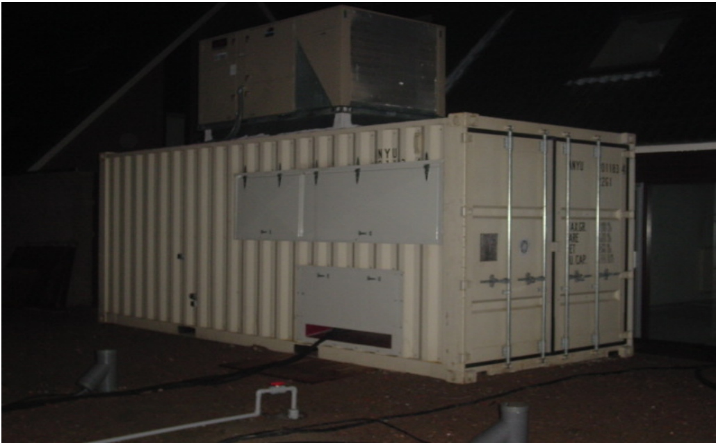
Six-Phase Heating Power Supply Unit (PSU)
